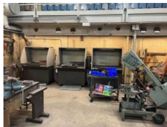
The grinding stations at the welding department.
